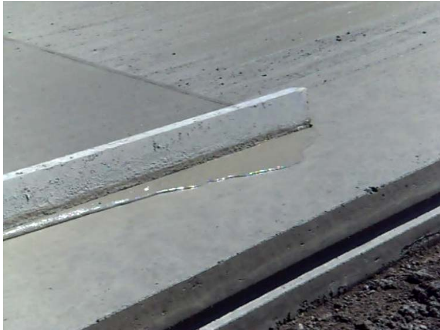
Figure 6. Slab Surface Tempered During Paving Operations.
