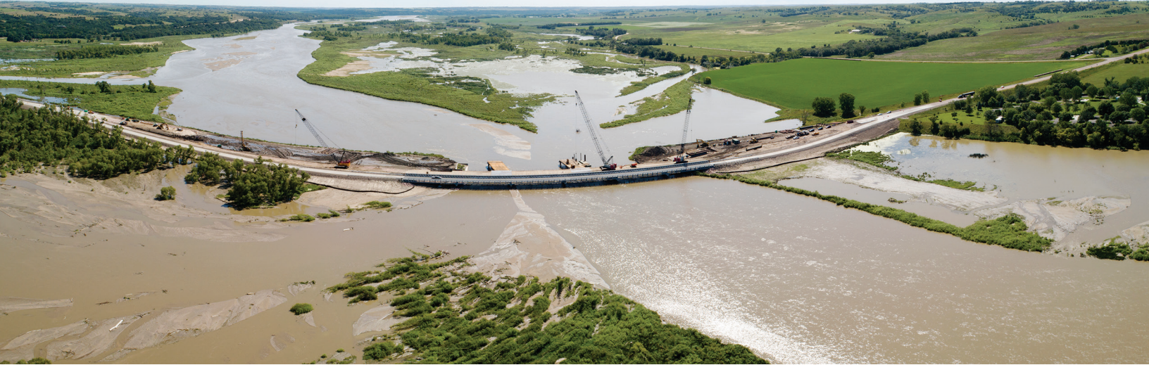
Work on the new bridge, next to the temporary bridge, is underway on Hwy. 12 west of Niobrara.
