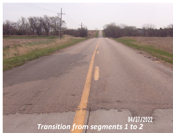
Figure 4: Change from Segment 1 (Reconstructed Good Condition Pavement) to Segment 2 (Poor Pavement within Project Area)
