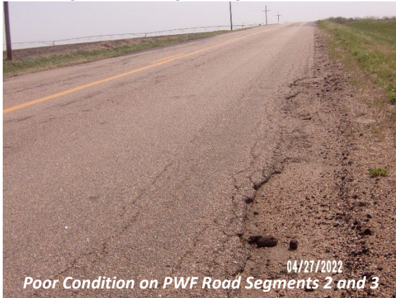
Figure 7: Road Edge Damage on PWF Road
