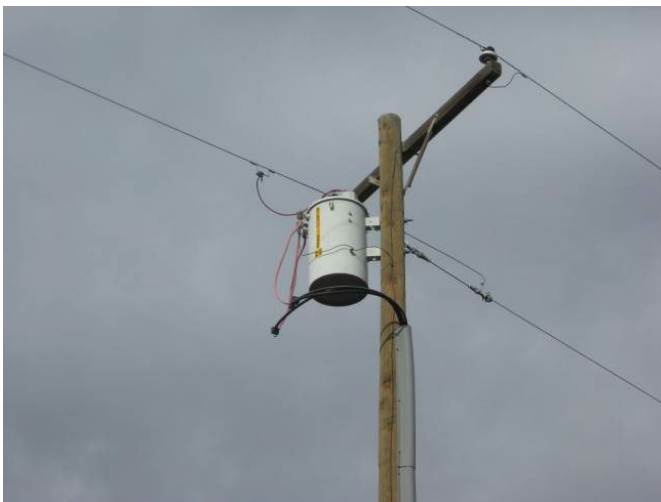
Pole-mounted electrical transformer in highway right-of-way.
