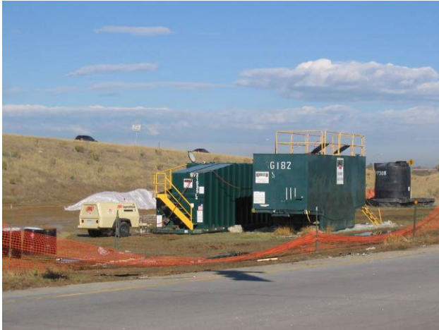
Baker remediation tank in highway right-of-way.
