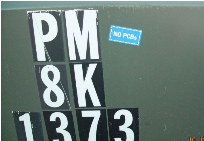
Pad-mounted electrical transformer.
