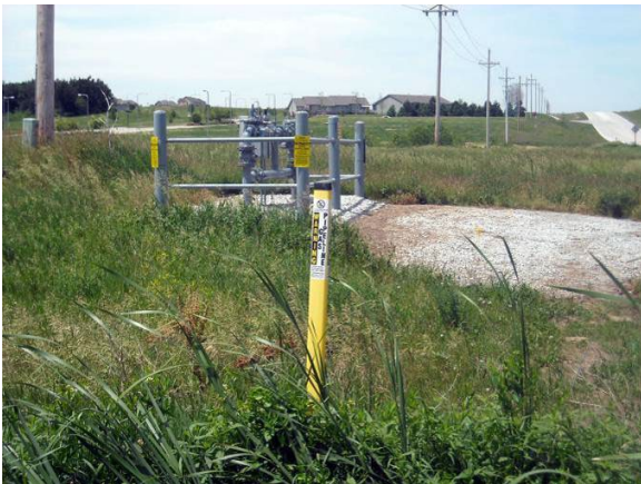
Gas line marker and regulator (background).
