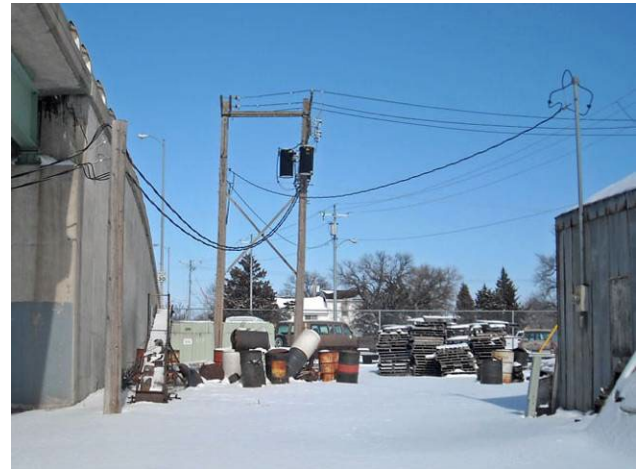
Pole-mounted electrical transformers. (Also note drums in bottom half of picture).
