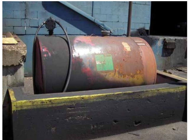
Typical used oil AST, with secondary containment in a concrete structure.
