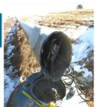
High Mast Tower Failure (Milford, NE, January, 2018)
