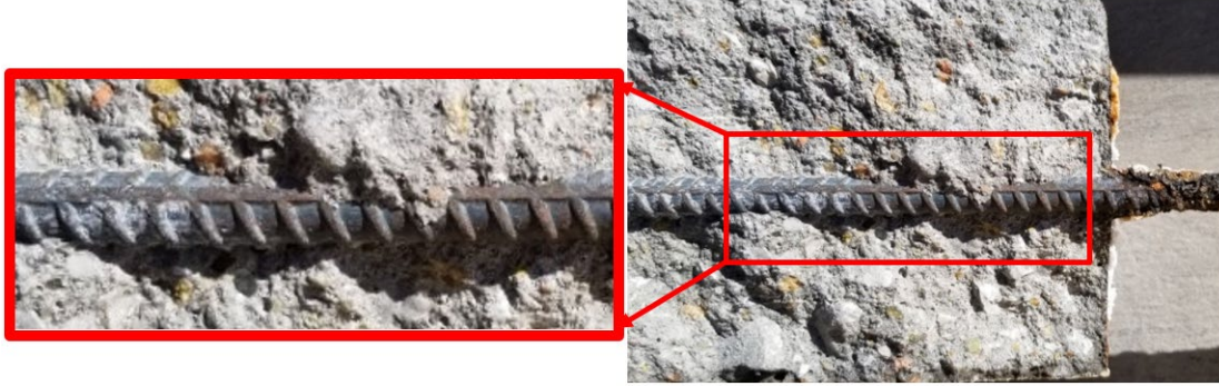
Figure 27. Specimen B- Day 132 condition verification: Very mild corrosion build-up on the rebar
