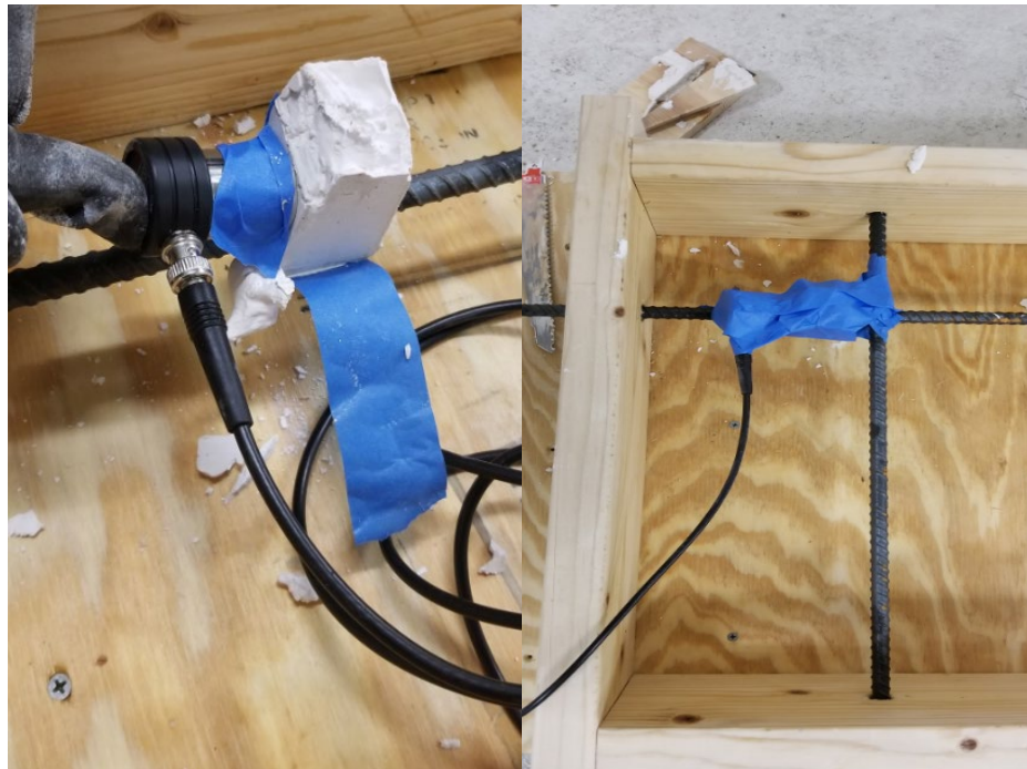
(a) (b) Figure 37. Sensor-to-rebar attachment: (a) sensor attached to the rebar using gypsum; (b) the sensor shown in (a) is wrapped using duct tape
