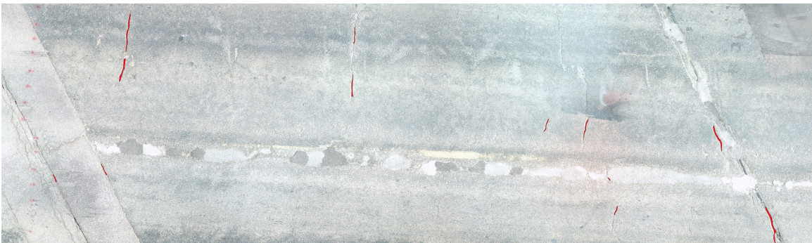
(b) Closeup view of the left top corner with cracks detected on Bridge S075 17596 (asphalt overlaid concrete deck)
