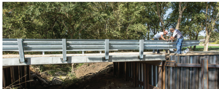
Thayer County bridge before and after reconstruction. Information about the County Bridge Match Program (CBMP) and the list of selected bridges is available at: dot.nebraska.gov/projects/tia/bridge-match/ .
