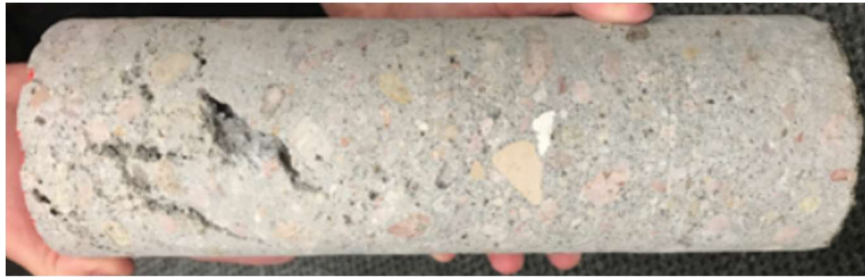
Figure 1 Air void in a cored concrete pavement sample
