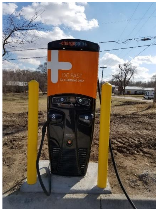
Figure 7.1 Location and the actual DC fast charger installed at Ashland
