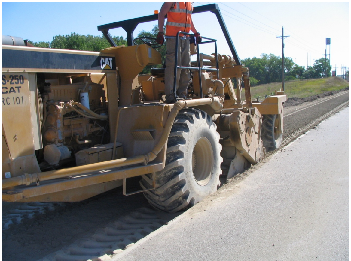
Figure 10: Soil Stabilizer SS-250 Caterpillar
