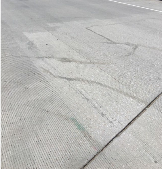
Figure 1.1 Early-age shrinkage cracks in bridge decks
