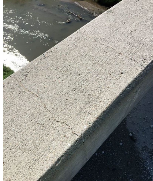
Figure 1.2 Early-age shrinkage cracks in bridge rails
