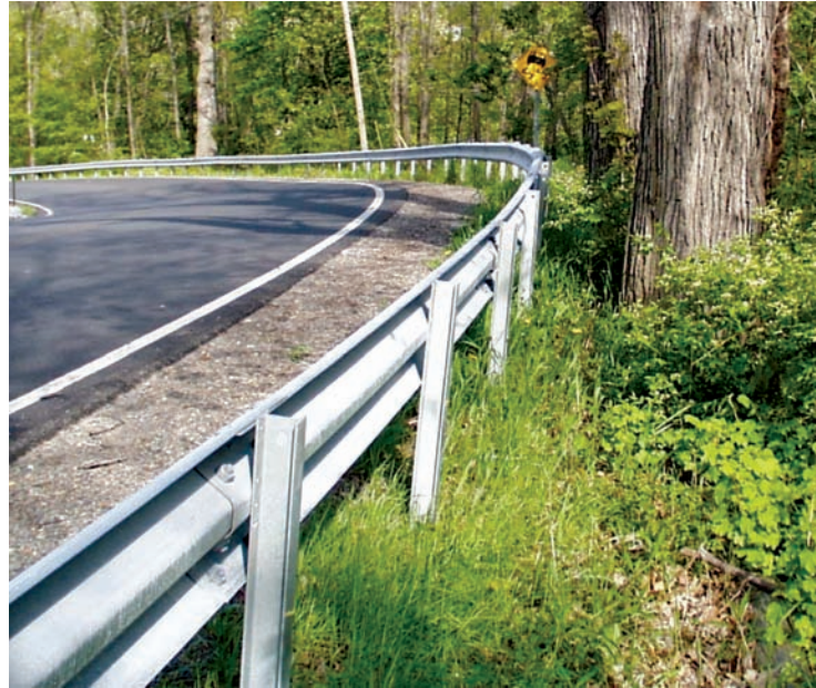
Figure 20 - Insufficient deflection distance
