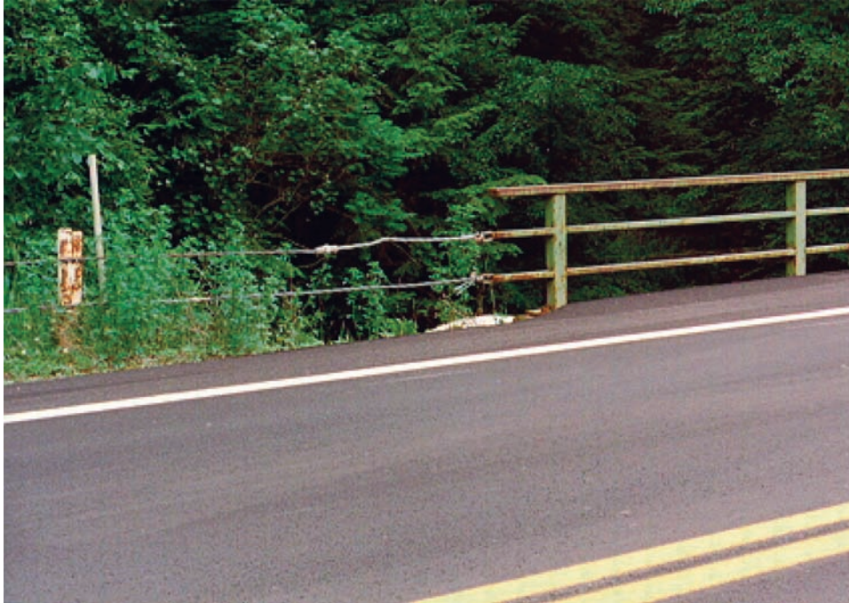
Figure 21 - Poor rail type transition
