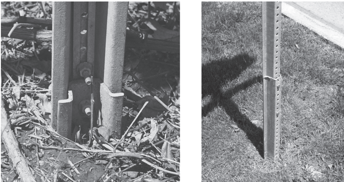
Figure 12 - Properly (left) and improperly (right) installed signposts
