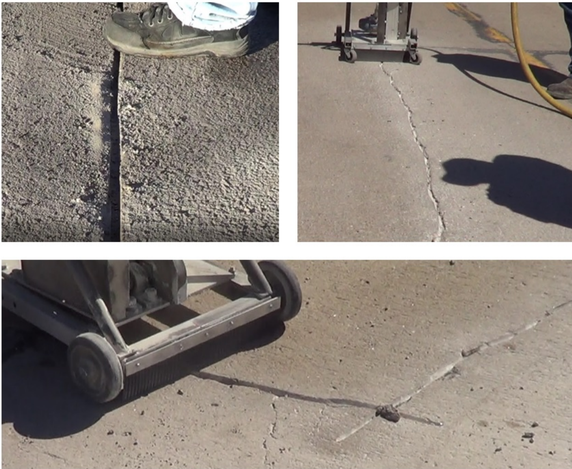
Figure 4.4 Cracks routed by CRD in concrete pavement
