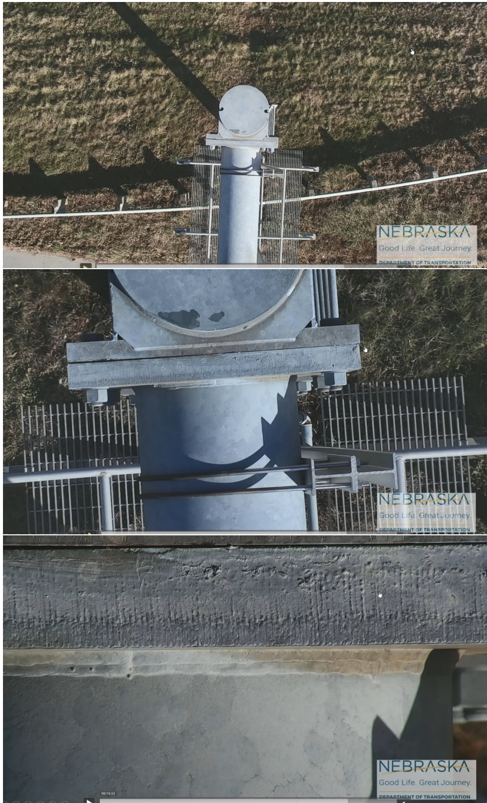
Figure 5 Image acquired in the inspection of the cantilever sign structure to examine welds and brackets for signs of rusting and spalling (top) and zoom in detail of the same image (center and lower).
