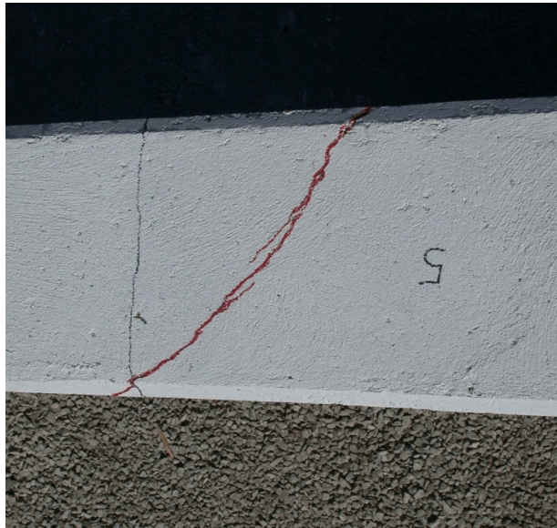
Figure 33. Open Concrete Bridge Rail Damage, Test NIT-1
