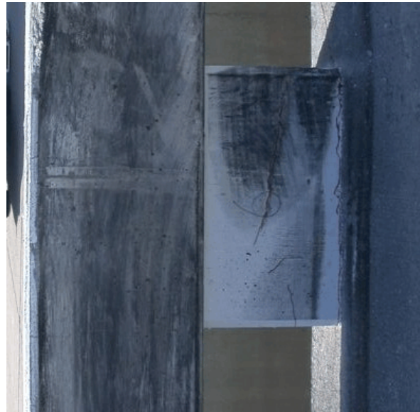
Figure 31. Open Concrete Bridge Rail Post Damage, Test NIT-1
