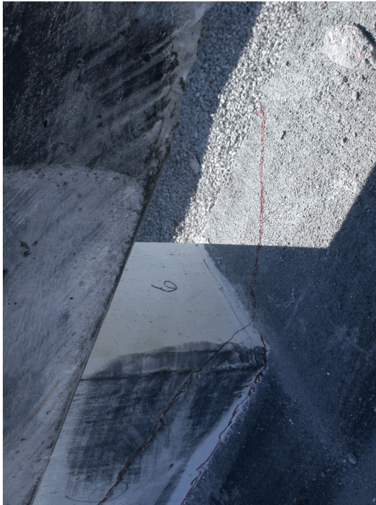
Figure 35. Bridge Deck Damage Around Post No. 6, Test NIT-1
