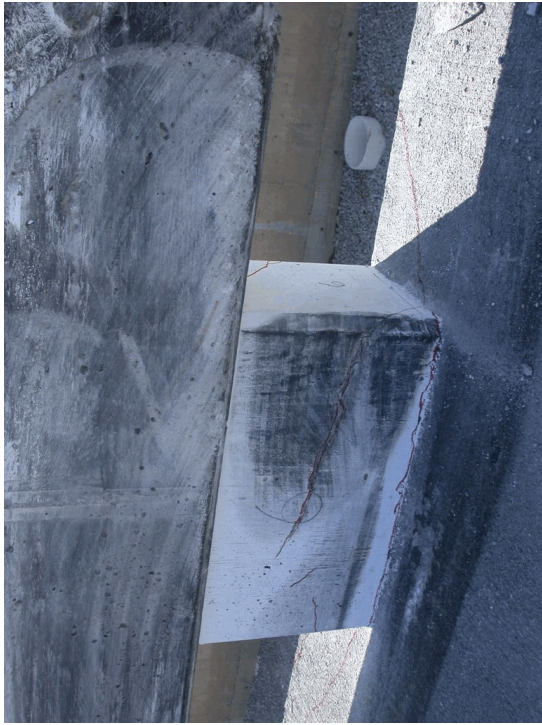
Figure 30. Open Concrete Bridge Rail System Damage, Test NIT-1
