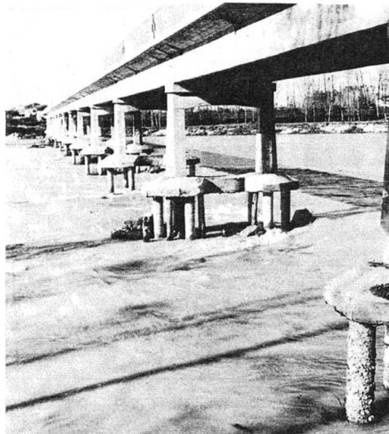
Figure 2.7 Degradation leads to bridge failure (after Galay, 1983)
