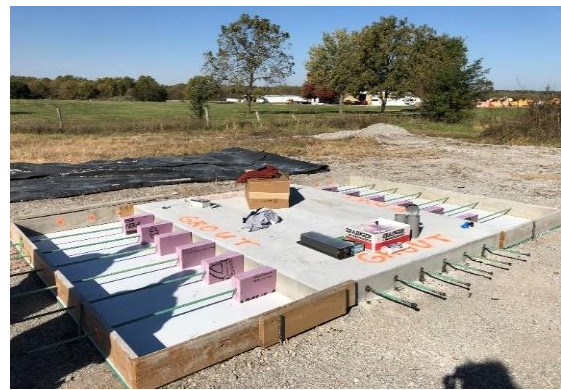
Figure 4 - The research slab awaiting placement of PR concrete. 18-inch bars were left exposed, while the 6-foot bars were embedded in the PR concrete. The pink foam inserts serve as a buffer to prevent sawing into the 47BD slab.
