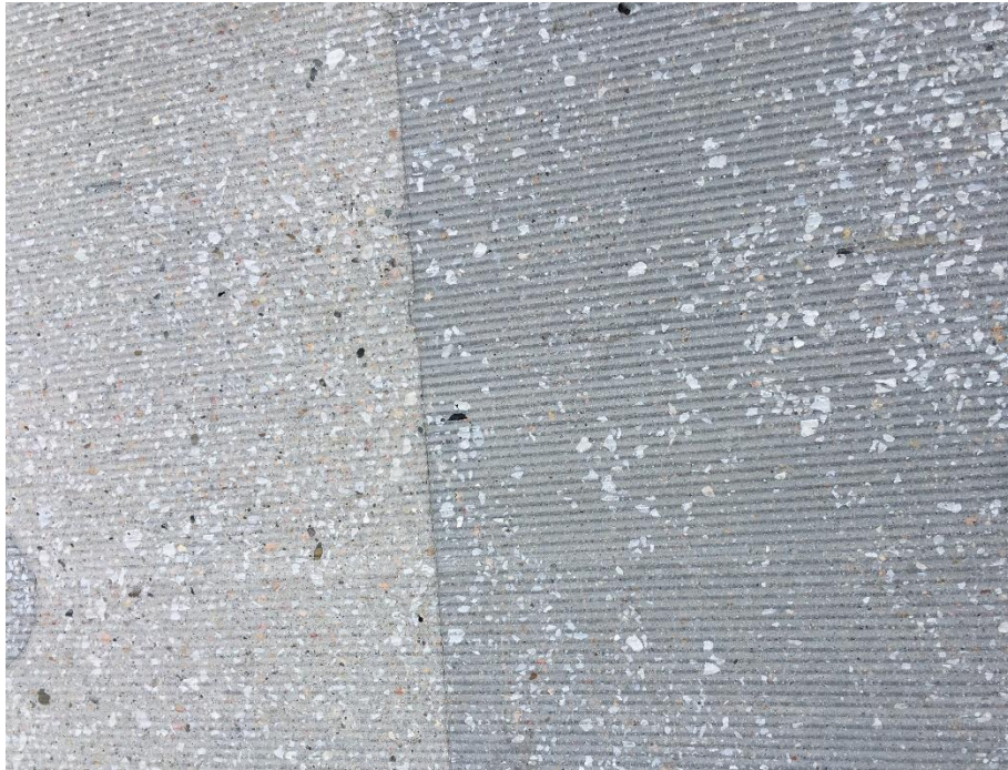
FIGURE 2.19 No cracking at the north anchorage blocks of precast concrete deck
