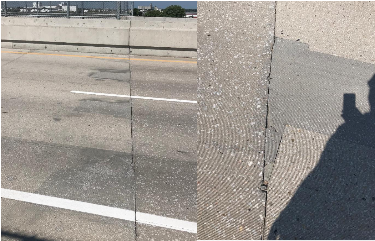
FIGURE 2.28 North (left) and south (right) PT anchorage blocks of the precast deck
