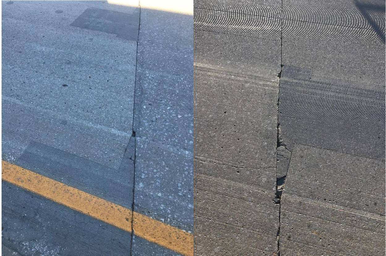
FIGURE 2.23 North (left) and south (right) PT anchorage blocks of the precast deck
