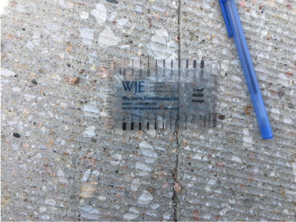
FIGURE 2.15 Measurement of the crack width at the intermediate pier joint
