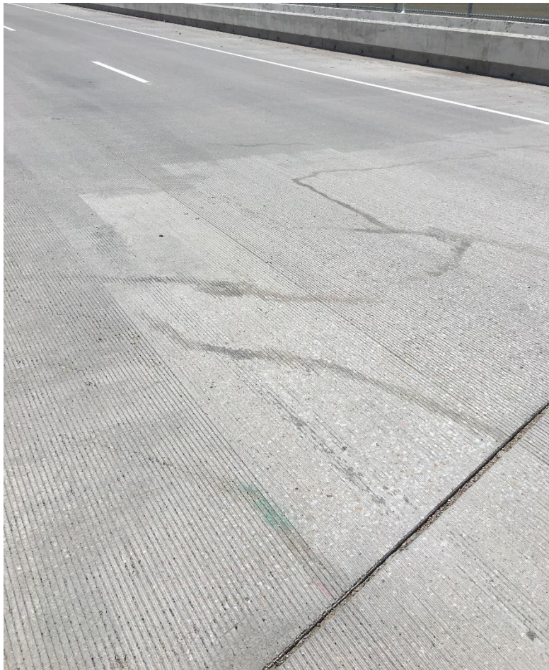
FIGURE 2.11 Diagonal cracks at the end of the skewed cast-in-place concrete deck
