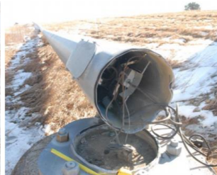
High Mast Tower Failure (Milford, NE, January 2018)
