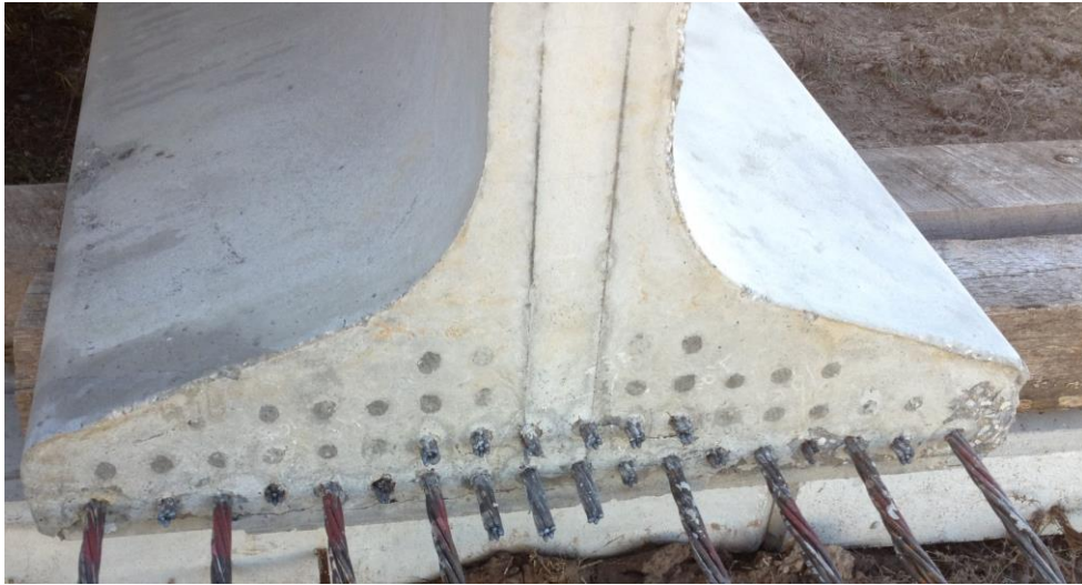
Figure 9: Photos of end zone of the 110 ft long girder (top left) ,end zone of 140 ft (top right) long girder, and between strands in the 110 ft long girder (bottom)
