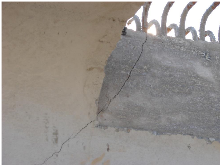
Figure 10: Cracking at girder ends where flanges are recessed.
