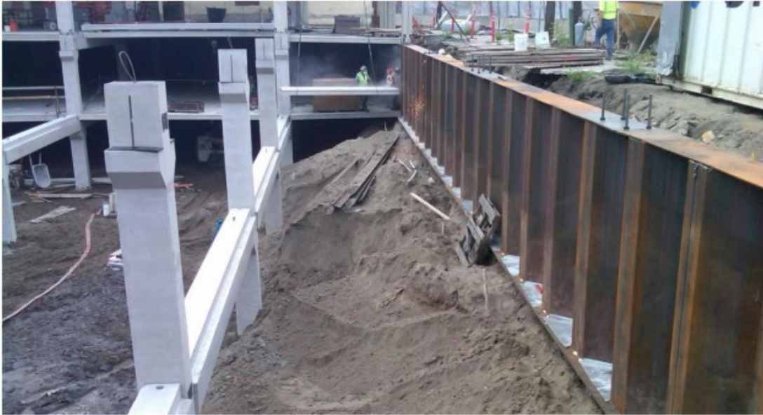
Figure 2.13 An example of sheet piling as a permanent foundation (with a temporary soil berm) for the construction of below-grade precast concrete framing (Underwood, 2020).
