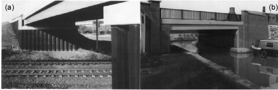
Figure 1.5 An example of sheet pile abutment bridges in Europe. (a) Humber Road bridge (Immingham, UK), and (b) Canal bridge (Stoke-on-Trent, UK). Images are from Yandzio (1998).
