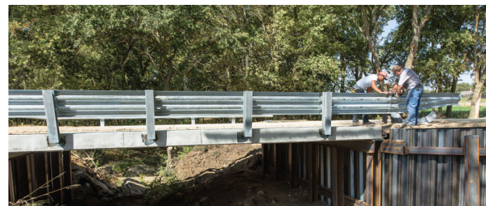
Thayer County bridge before and after reconstruction. Information about the County Bridge Match Program (CBMP) and the list of selected bridges is available at: dot.nebraska.gov/projects/tia/bridge-match/ .
