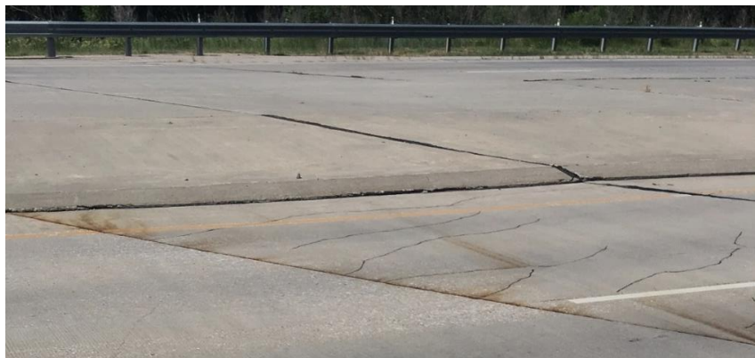
Figure 1.1: Cracking of bridge approach slabs
