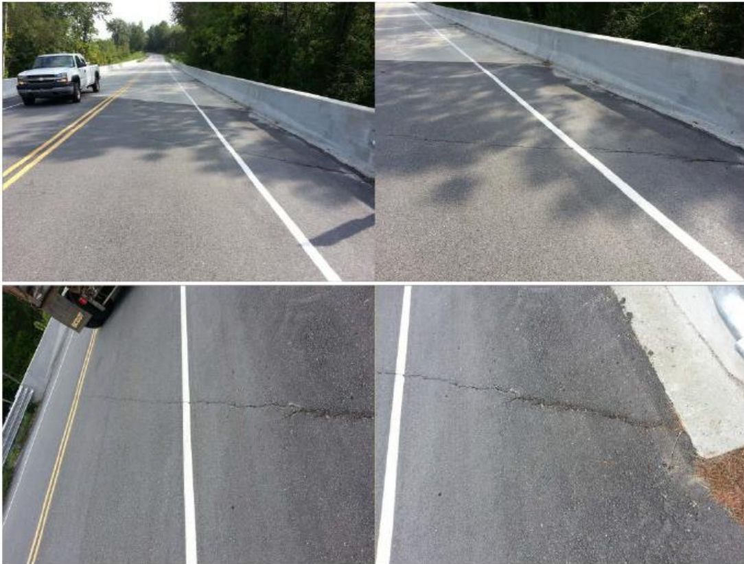
Asphalt cracking at paving end of the approach slabs
