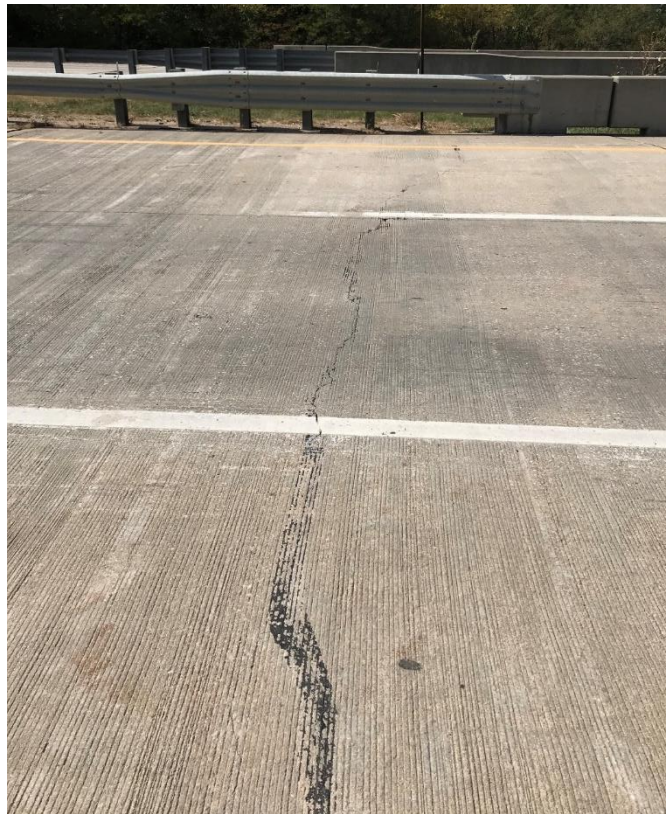
Figure 3.8: Turkey Creek bridge approach slab and paving section cracking
