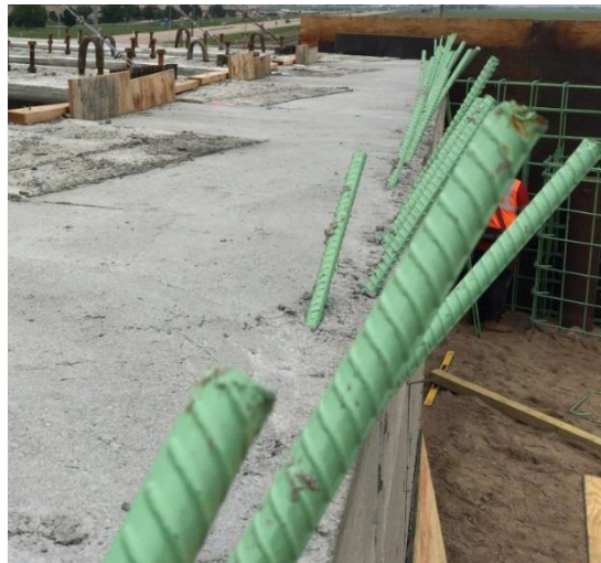
Figure 4.23: Current practice of using #6 @12 in. dowels to connect approach slab at the abutment
