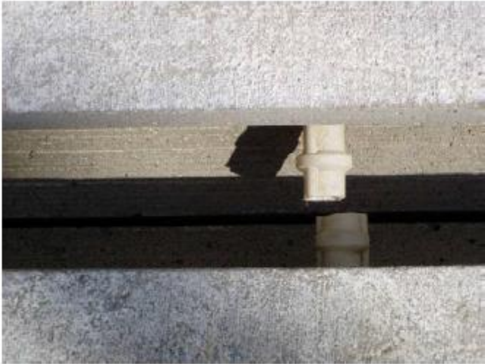
Misalignment of ducts
