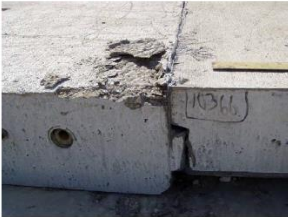
Damage at panel corners
