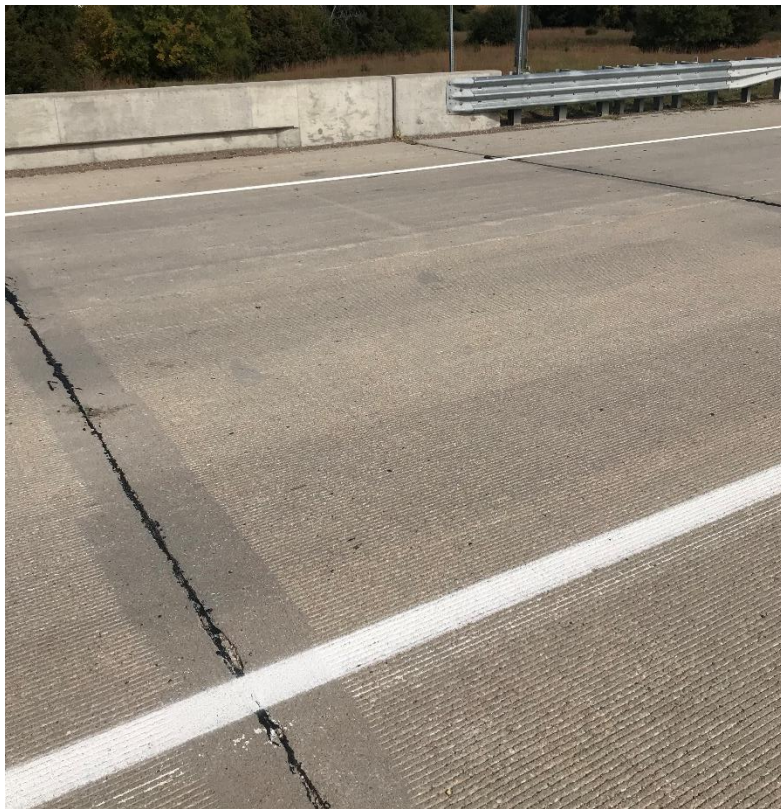
Figure 3.6: Little Sandy Creek bridge approach slab and paving section cracking
