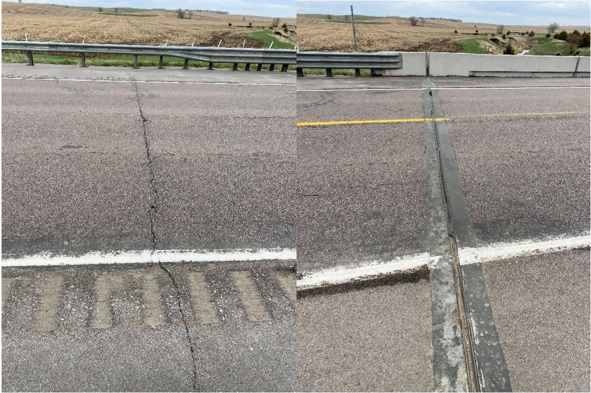
Asphalt cracking at the end of paving section (left) and expansion joint (right)
