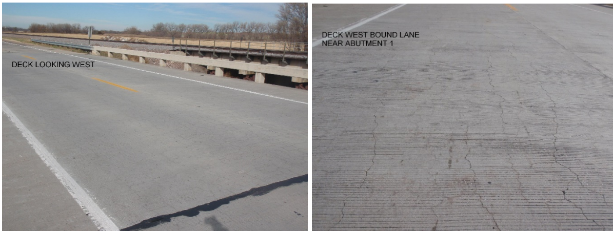
Figure 1. Examples of bridge deck cracking (photos from NDOT Bridge Inspection Database)
