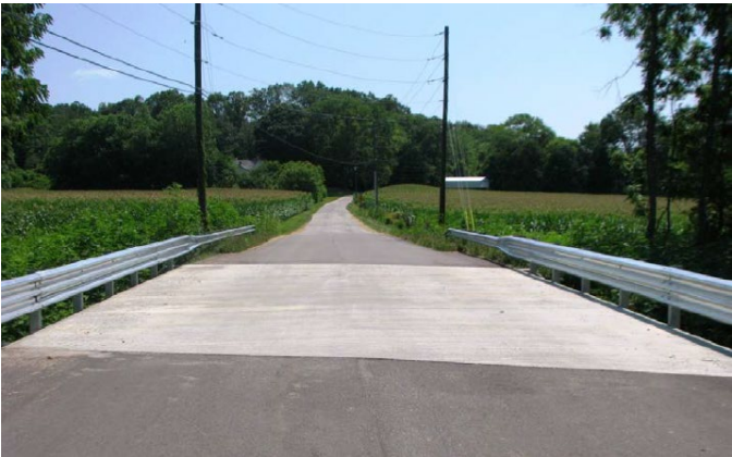
(b) Internally cured bridge deck with no cracks
