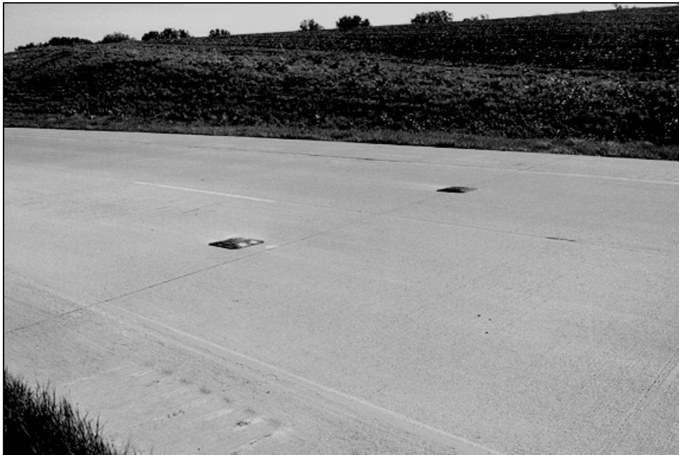
Figure 4.3 NC-97 Detectors Installed Under Protective Covers on Expressway
