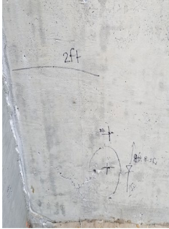
(b) marking the center of each pressure cell on the abutment walls
