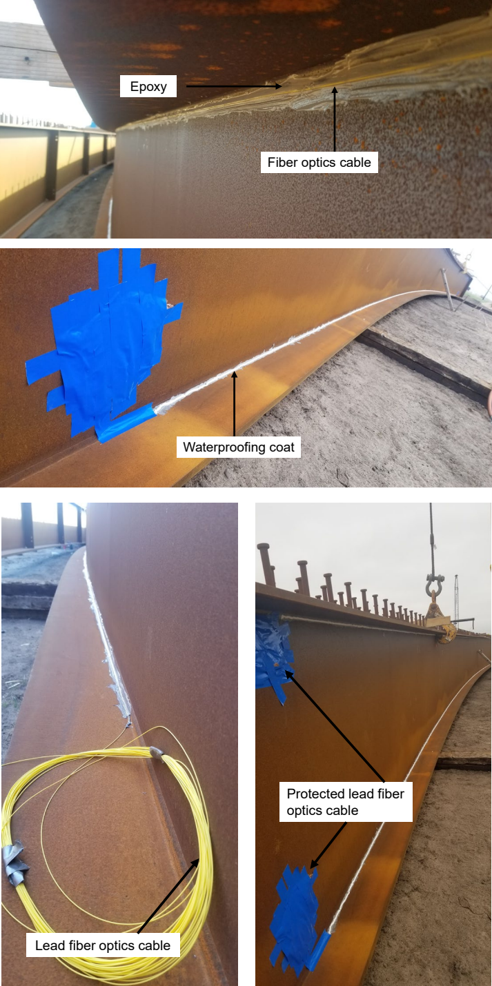
Figure 3.40: Fiber Optic Cable Installation on the Girder with Epoxy and Waterproof Coat, and the Lead Cable Protected in Plastic Bags for Future Splicing Task
