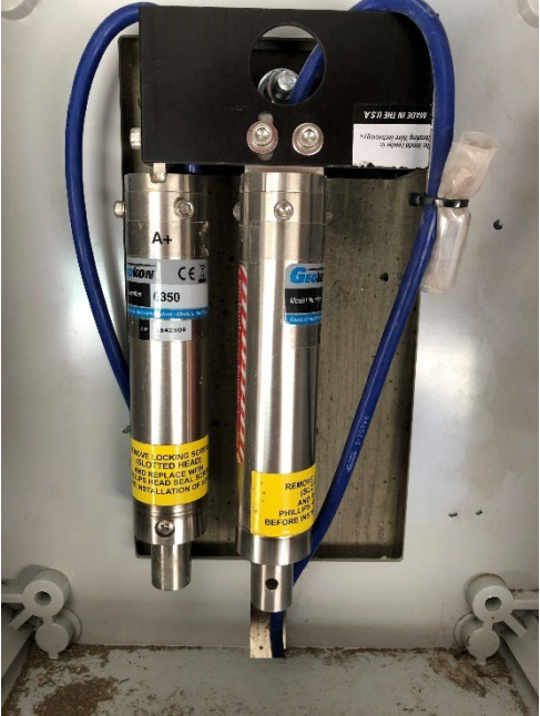
(a) longitudinal and lateral tiltmeters
