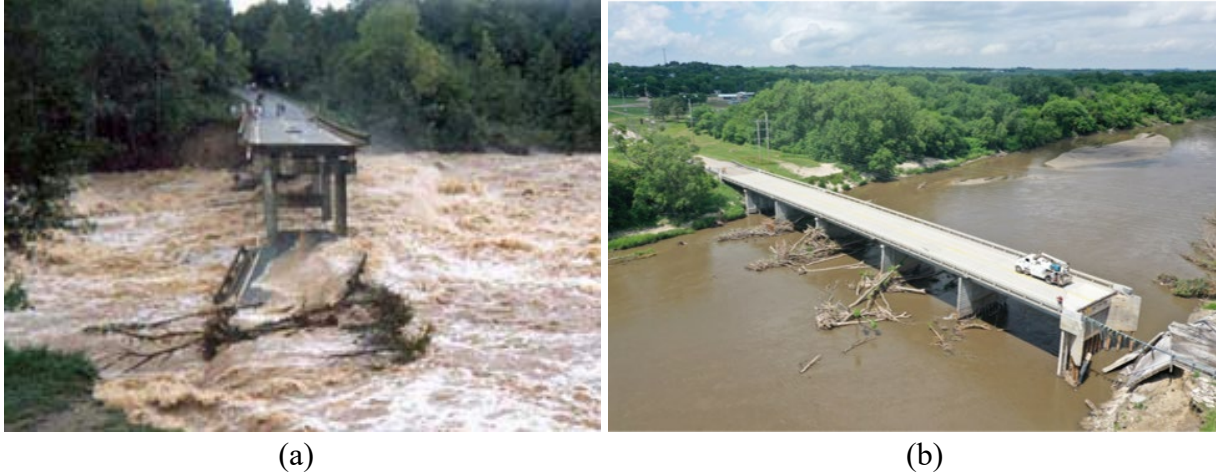
Figure 2.1: Bridge failure due to scour (a) Enoree river bridge (photograph by Michael Hall, 1995), (b) Stanton County bridge (photograph by Richard Wood, 2019).
