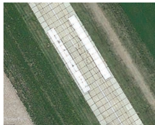
Pavement Distresses on runway 14/32
