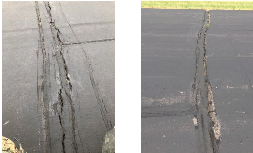
Transverse runway cracks at Bloomfield
